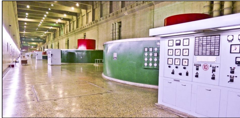
Figure 4.8 - Generators inside a HEP Powerhouse (Tarbela dam)
