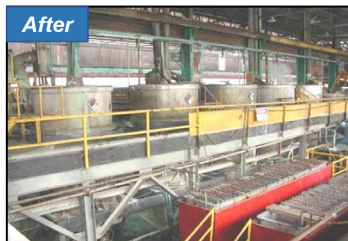
Copper sulfate cells to treat acidic solutions from copper refinery (c. 2004).
