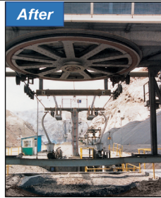
New cable car system for slag transport (2005).
